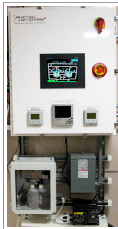
CMS System Control Station
