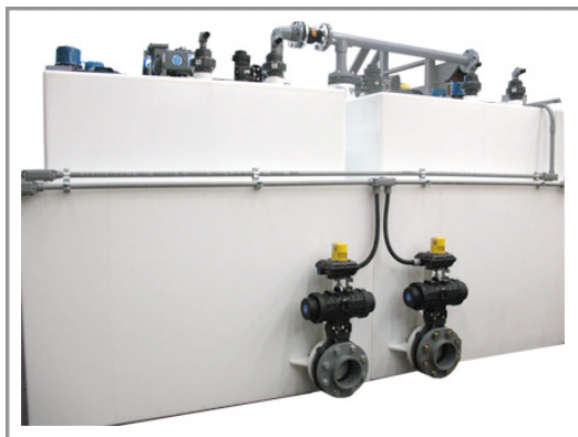
CMS System Tanks
